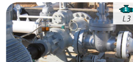
BOOSTER PUMP L3 AND L4
