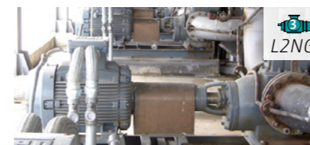
CRUDE TRANSFER PUMPS L2, L3 AND L4
