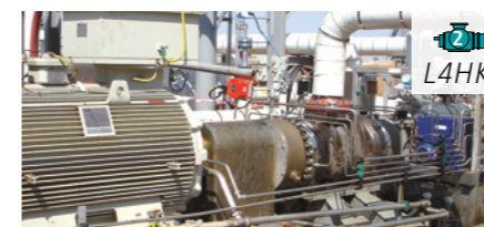
START-UP PUMPS L3 AND L4
